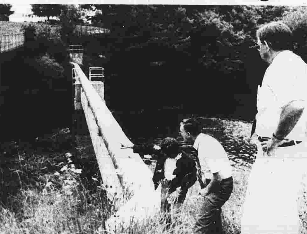
Republicans point out woes at Union Street Bridge this morning. From left, they are Directors Peter DiRosa and William Diana and state Sen. Carl A. Zinsner, a former director.
